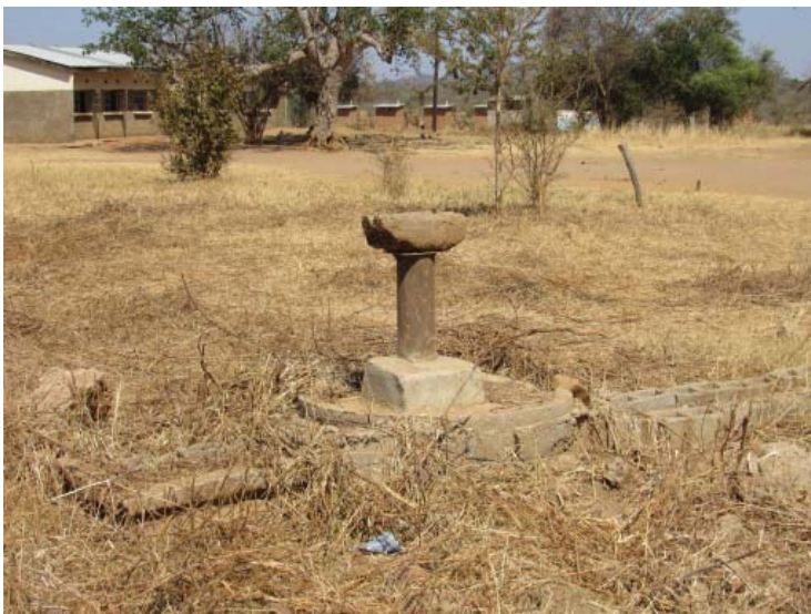
Water well found with no hand pump at Kachembele Community School
